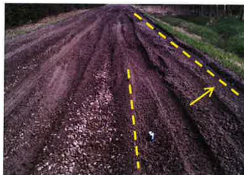
Fig. 2 Mountain View County Road damage caused by drilling rig move – rutting and road edge pushed out
