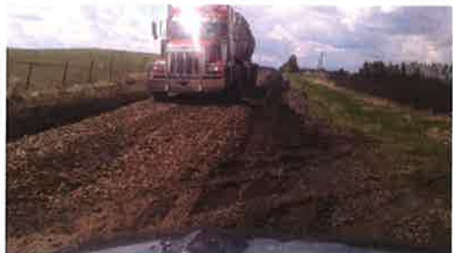
Fig. 6 Mountain View County Damage has required operator to lay pit run gravel in the centre to allow continued movement of trucks
